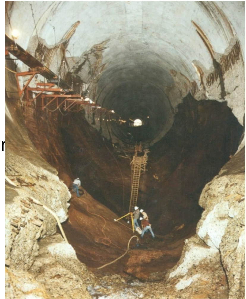
Damage to spillway following 1983
