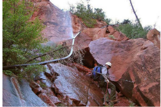
Leak along the Transcanyon Pipeline
