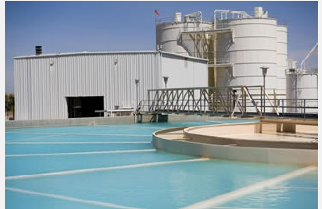
Yuma Desalting Plant - BoR
